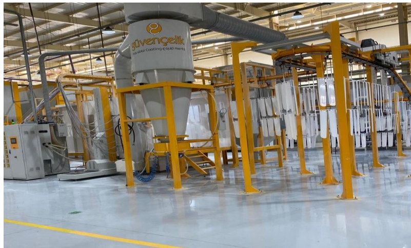
Fig. 10 Electrostatic painting plant
