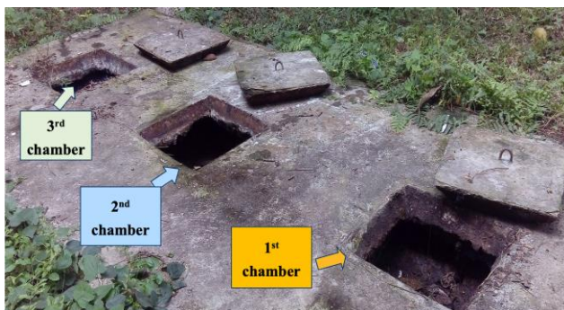
Fig. 2 The studied septic tank at KUET campus with three respective chambers.
