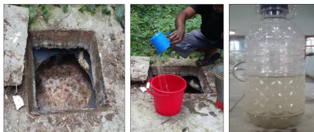
Fig. 3 The left side picture shows a 1st chamber of the septic tank, and the middle picture shows the collection of wastewaters from the 2nd chamber. Moreover, right side picture shows the sample of wastewater that was collected from the chamber of the septic tank
