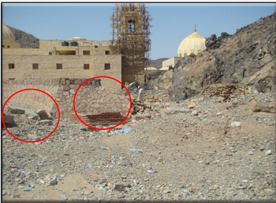
Part of the wall of Sheikh Al-Shazly Mosque collapsed due to floods
