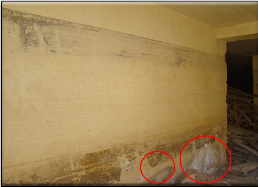
The walls of the storeroom of Sheikh Al-Shazly Mosque were affected by flood waters
