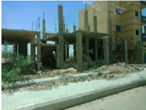
Figure 11: Destruction and Incompleteness of the house.
