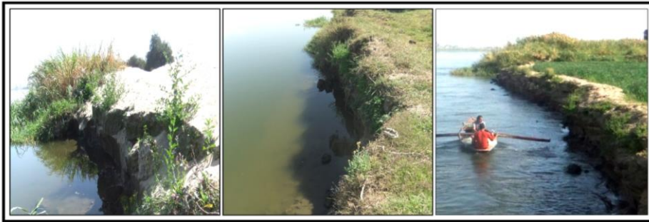
Figure 16: The Impact of Erosion Process on the Banks of the Nile Stream in the Abnub Area
