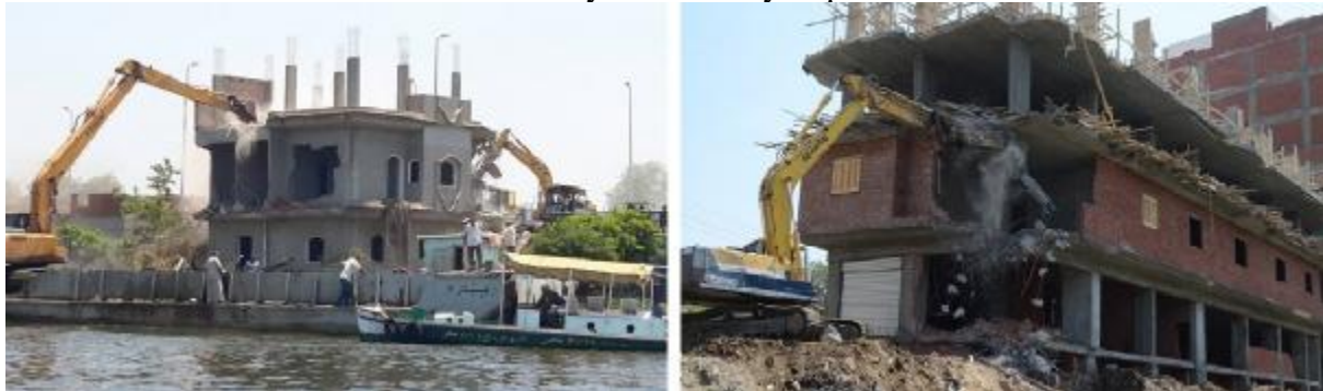
Fig (8) Removing the encroachments from the agricultural land and from the banks of the rivers
