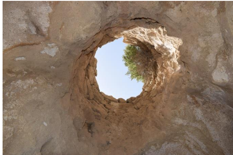
Pic. 7. The nozzle of the shaft for receiving rainwater.
