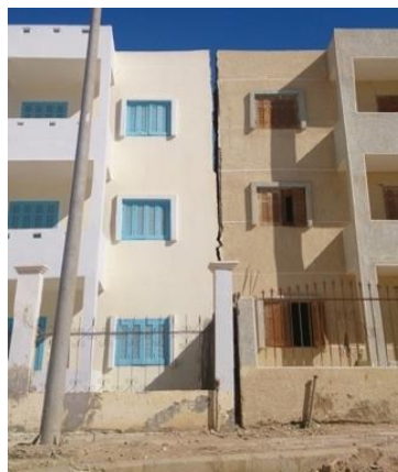
Figure 5 Example of structural problems of Ibny Baitak model (pictured in July 2023) [39].
