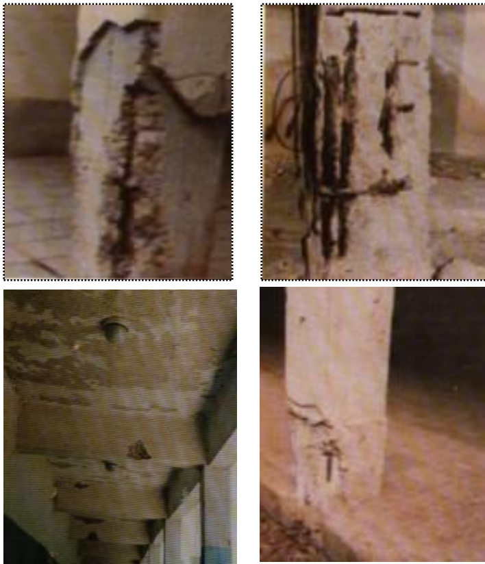
Figure (18) a,b,c,d : From the results of the visual examination of the defects of the school, we note the presence of cracks in the concrete slabs, columns and beams ( Source: Author ).
