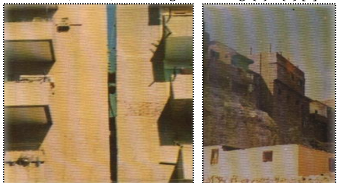
Figure (3): A clear slope in one of the buildings Figure (4) : Buildings on the edge of a mountain are susceptible to sliding (Source: Author).
