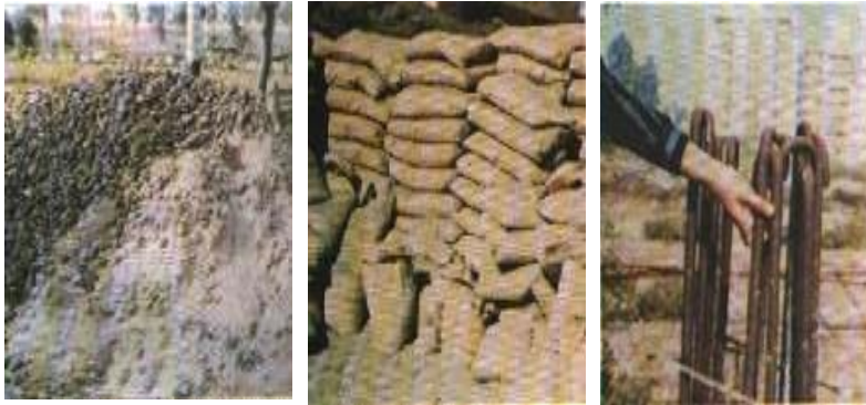
Figure (5): bad storage of gravel Figure (6): bad cement storage Figure (7): Steel reinforcement with a high percentage of rust (Source: ref. [3]).
