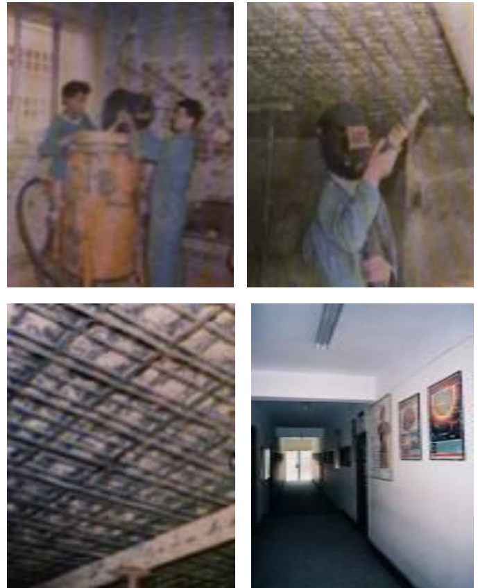
Figure (19) a, b : covering the slab with a layer of concrete with a concrete spray gun Figure (20) a, b : adding a bottom steel meshes to the slab & the Concrete slab after maintenance and rehabilitation ( Source: Author ).
