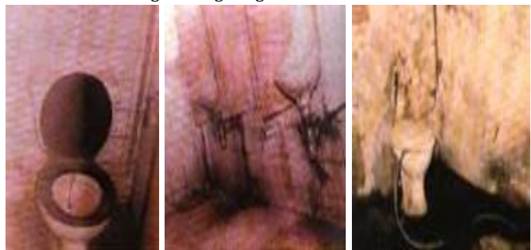
Figure (12) a, b, c: Poor condition of plumbing devices and bathrooms, which requires maintenance work (Source: ref. [13]).
