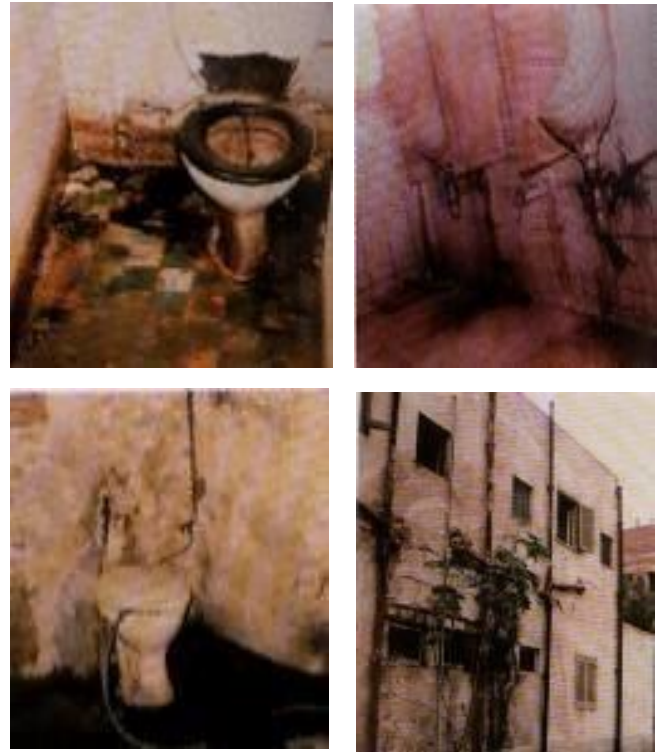
Figure (24) a, b, c, D: Visual inspection and the application of maintenance checkups proved the poor condition of the bathrooms, which required the complete replacement and change of the bathrooms (Source: Author).
