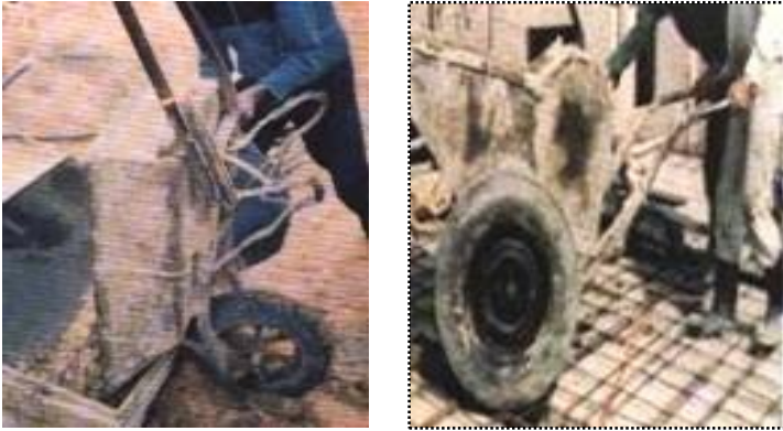
Figure (10): Wrong gravel calibration method
