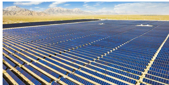
Figure 5. Solar (PV) Independent Power Product, Aswan- Egypt
