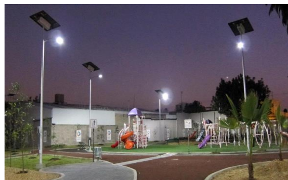
Figure 14. Street solar lights
