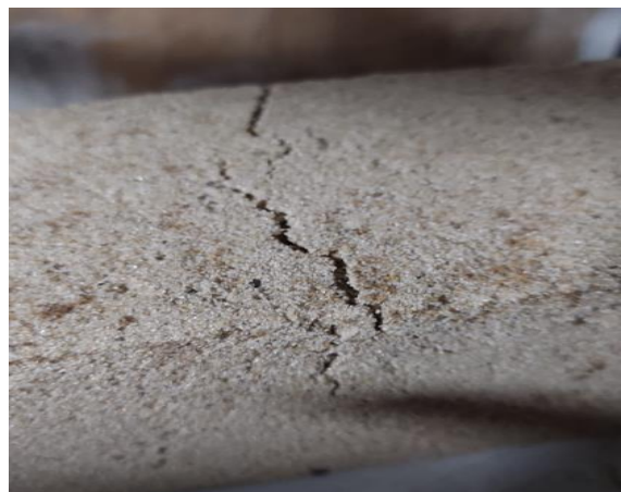
Figure 18 Zoom on Beam on failure. 30% of SS21
