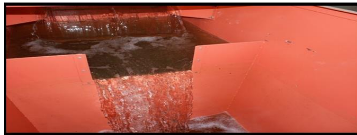
Figure (2) Measuring weir
