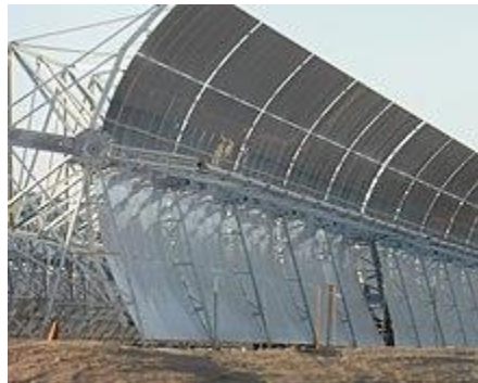
Fig. 7 Parabolic trough at a plant in Harper Lake, California
