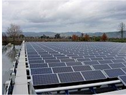
Fig. 6 Floating photovoltaic on an irrigation pond
