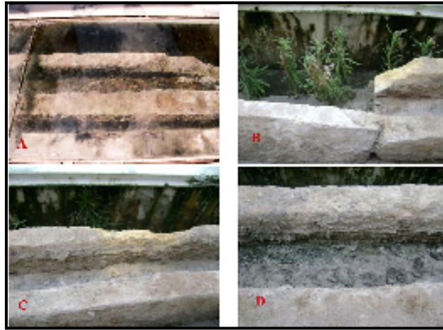
Fig. 4 Shows the degradation phenomena of the water duct. (A) Shows the discoloration of stone surface due to the accumulations of colored stains of microorganisms. (B) Shows the vascular plants growing in the bottom of the water duct. (C) Shows the eroded edges of the water duct due to the exfoliation and detachment of the superficial layer. (D) Show the black crust accumulated on the stone surface
