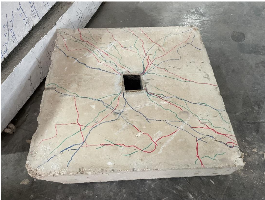
Fig. 10. Crack pattern of slab (S2).
