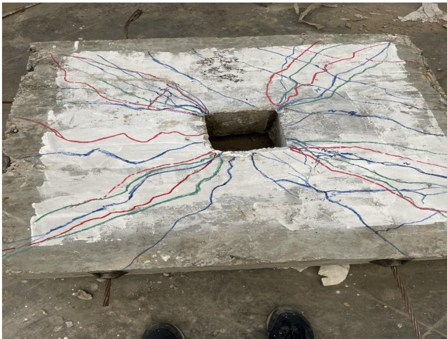
Fig. 12. Crack pattern of slab (S4).
