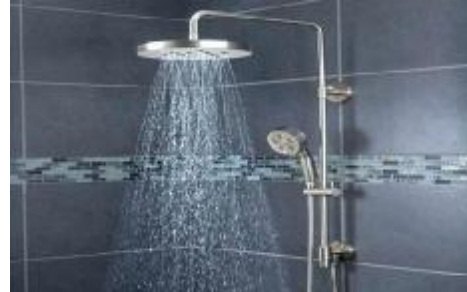
Figure 8: fixed and movable shower head Source: Guidelines for the Planning of Houses for Senior Citizens, 2007
