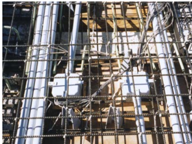
FIGURE 13. SENSORS EMBEDDED IN THE DECK OF TAYLOR'S BRIDGE [23].
