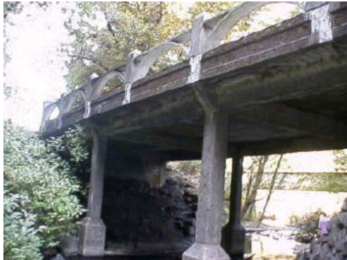
FIGURE 14 HORSETAIL BRIDGE BEFORE STRENGTHENING.
