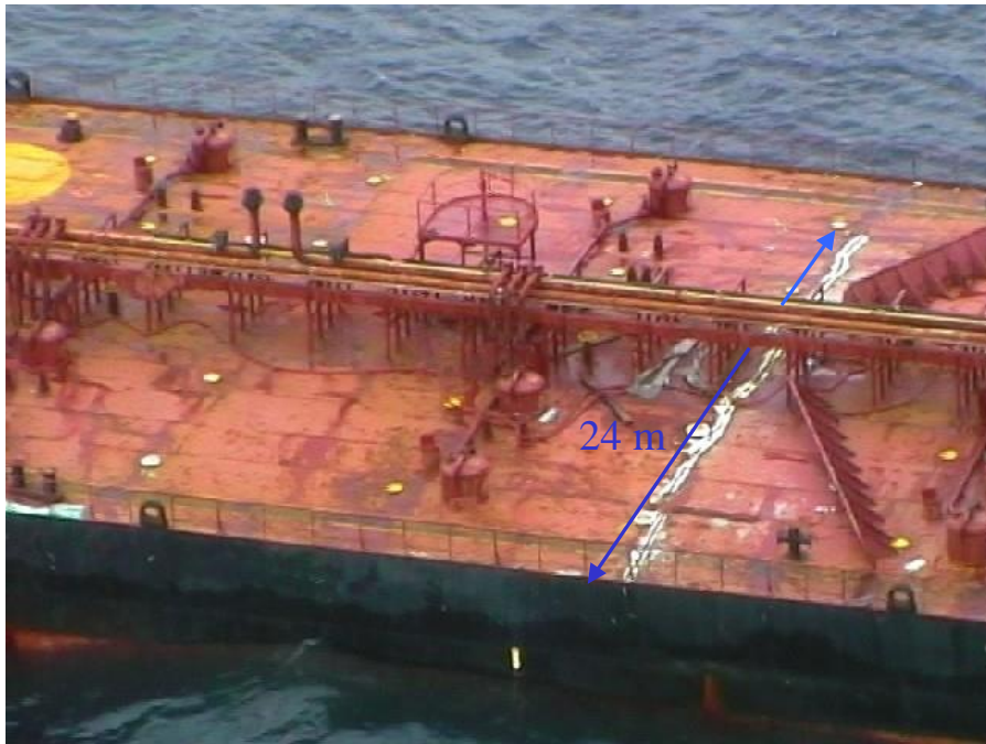
Figure 1 - Cracked deck in the tanker Castor
