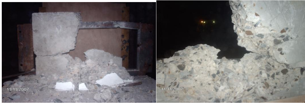
Damage in Front Face of plain concrete slab Damage in rear Face of plain concrete slab
