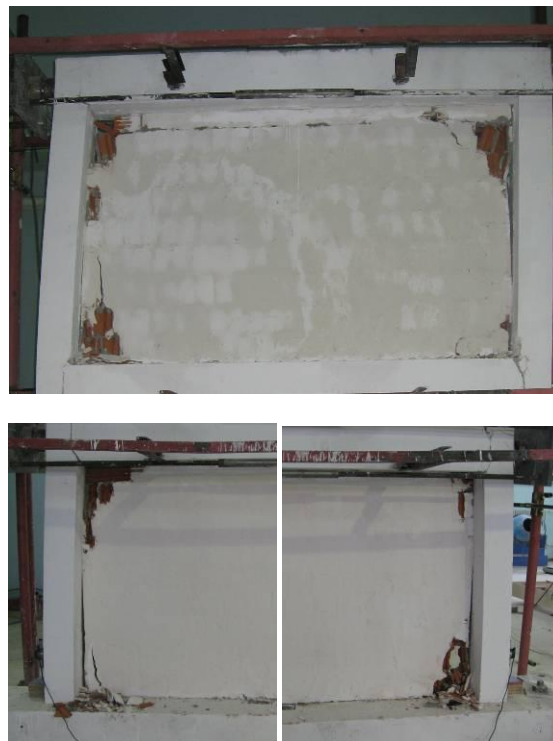
Figure (7) Failure modes of the wall portions
