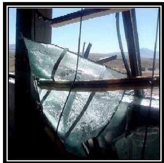
Fig. (6) View of the cable system after detonation
