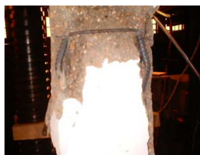
b) Failure of CR1
