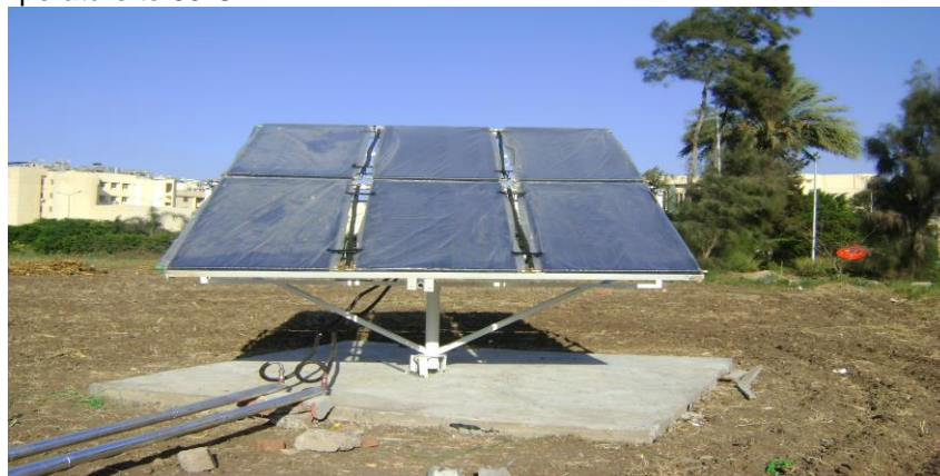
Fig. (2): Solar collector panel array, with a total surface area of 12.0 m 2 and mounted on a movable frame.
