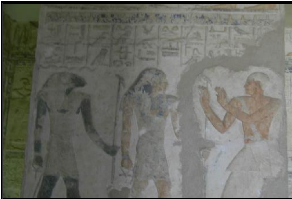
Figure 5. Restoration of diagonal fissure on a tomb wall in Beni Hassan.
