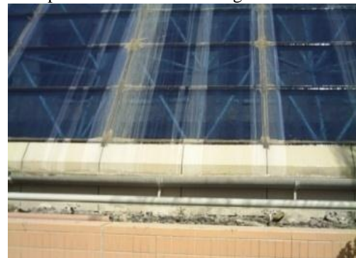
Fig (4) Water falls on curtain wall at city stars mall Source: Researcher
