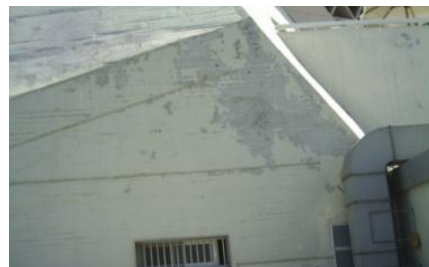
Fig (7) Cracks in the facades of the conference hall - Bibliotheca Alexandrina Source: Researcher
