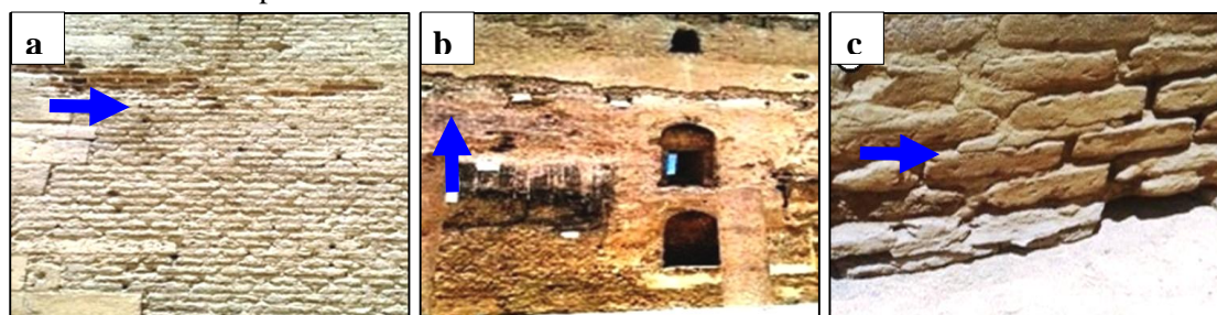
Figure (3-a,b,c) Shows different deterioration and degradation features affected the historical red bricks at the Red Monastery (the arrow refer to the N).
