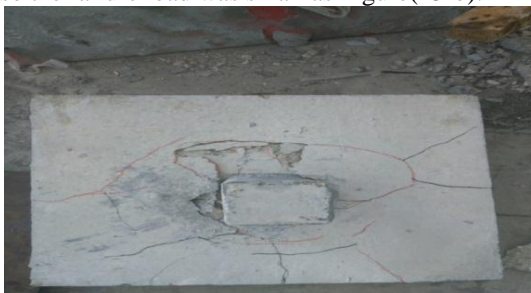
Figure (12): Shape of failure for slab S 21
