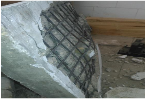
Figure(15-b): The crack pattern for slabs S4
