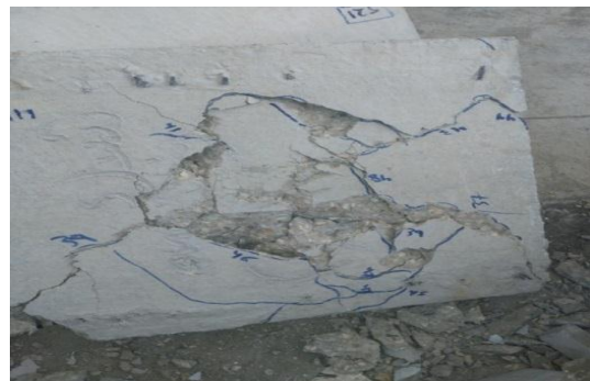
Figure (14): Shape of failure for slab S 23
