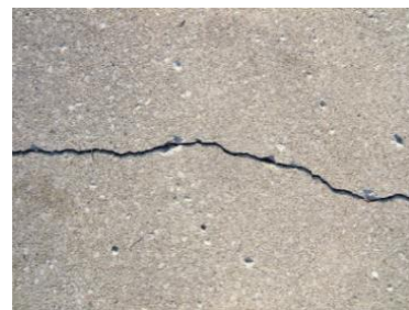
Figure 11: Actual image of crack
