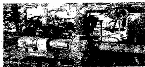
Photo (5) Feeding Water Pump
