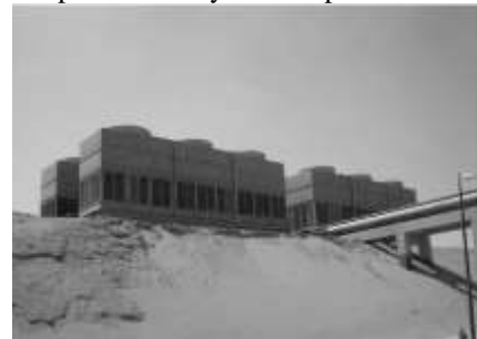
Fig. 15. Cooling towers at AUC's central utility plant.[36]
