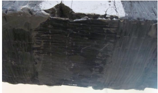
Fig. (6) Close view showing debonding and rupture of CFRP sheet of tested beam A0-S12
