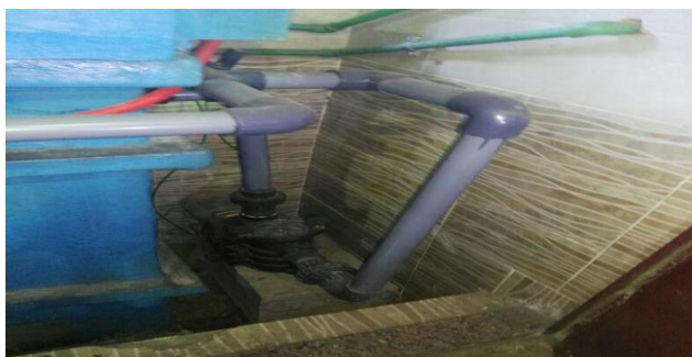
Fig. 2: Pump & inlet and outlet plumbing connections
