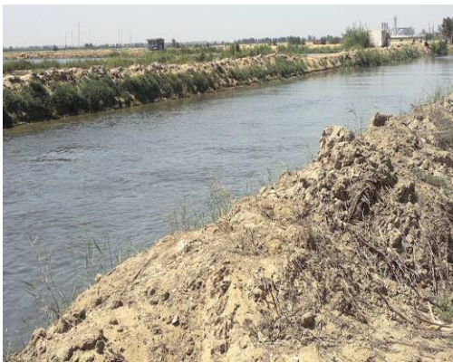
Fig. 9. The embankments failure along Mayo Canal
