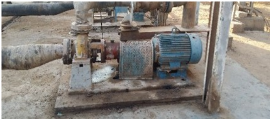
Fig. 5a: HP water pump201
