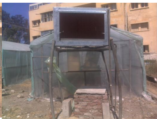
b- Evaporative cooling unit
