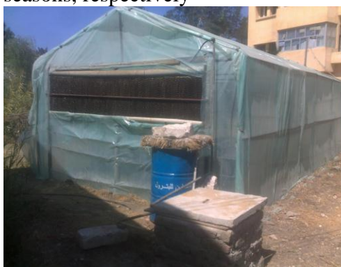
a- Fan-pad evaporative cooling system
