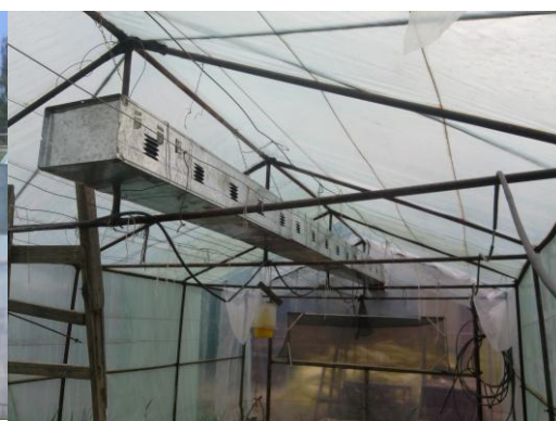
d- Perforated duct hanged across the greenhouse longitudinal axis
