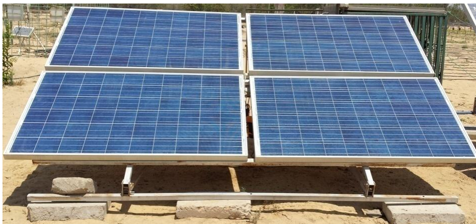
Fig. (1): NESL (PV) polycrystalline 240 W (4 modules).
