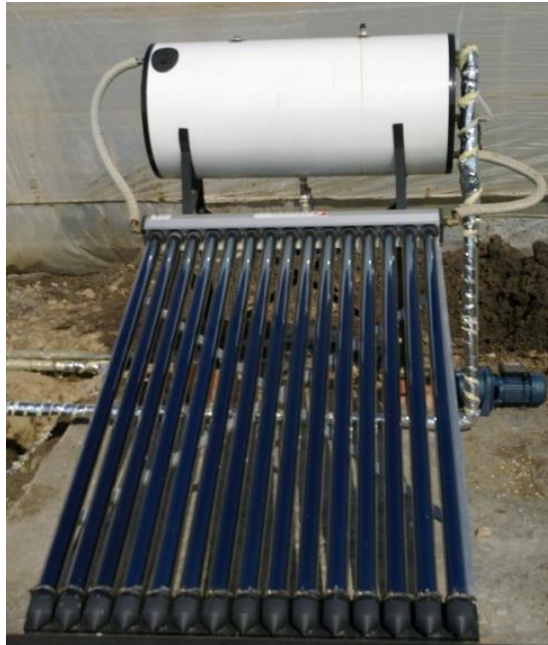
Fig. 2: Actual evacuated tube collector installation
