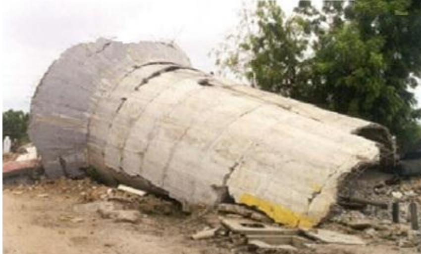
Fig.1 Collapsed elevated water tank in Bhuj 2001 earthquake
